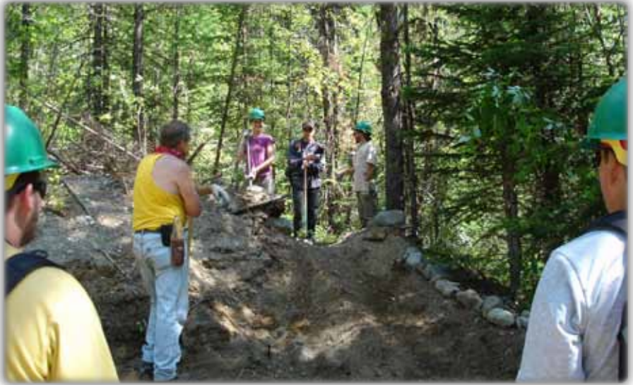
Volunteers repairing a road bar, meant to exclude illegal ORV use at a site of frequent ORV trespass in the Colville National Forest.
